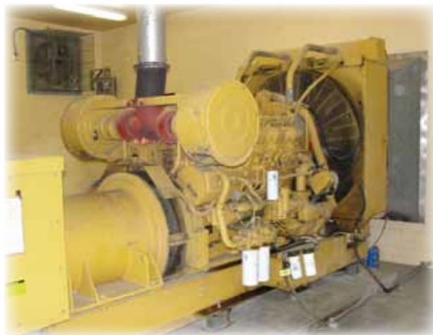
Generator with Cat 3508 engine
